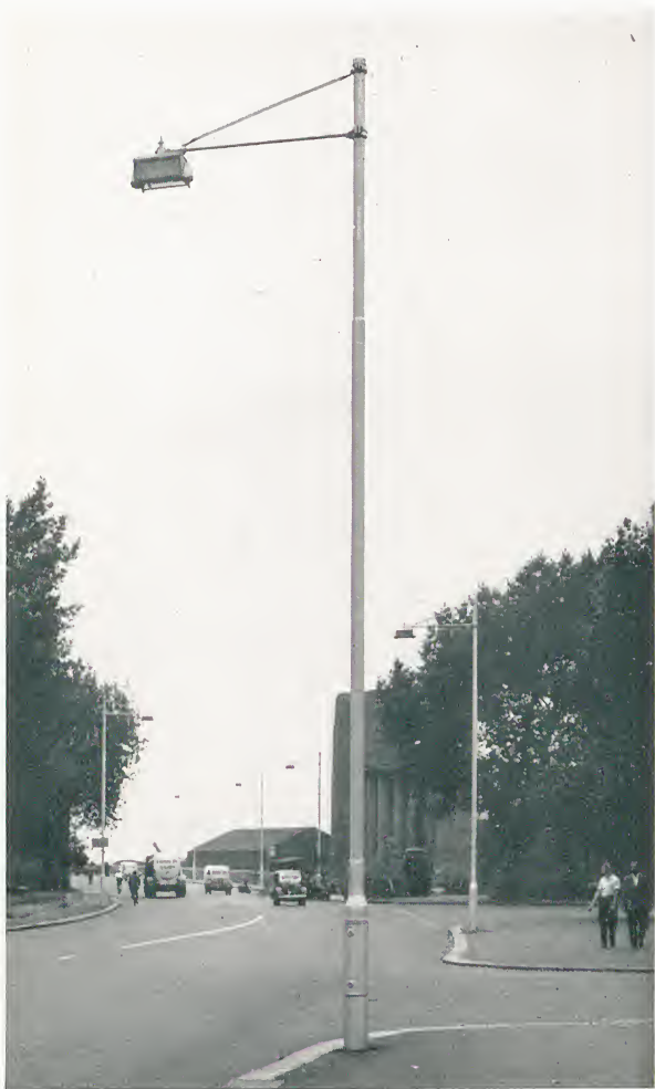
'S & L' tubular steel lighting columns having a mounting height of 25 ft.
